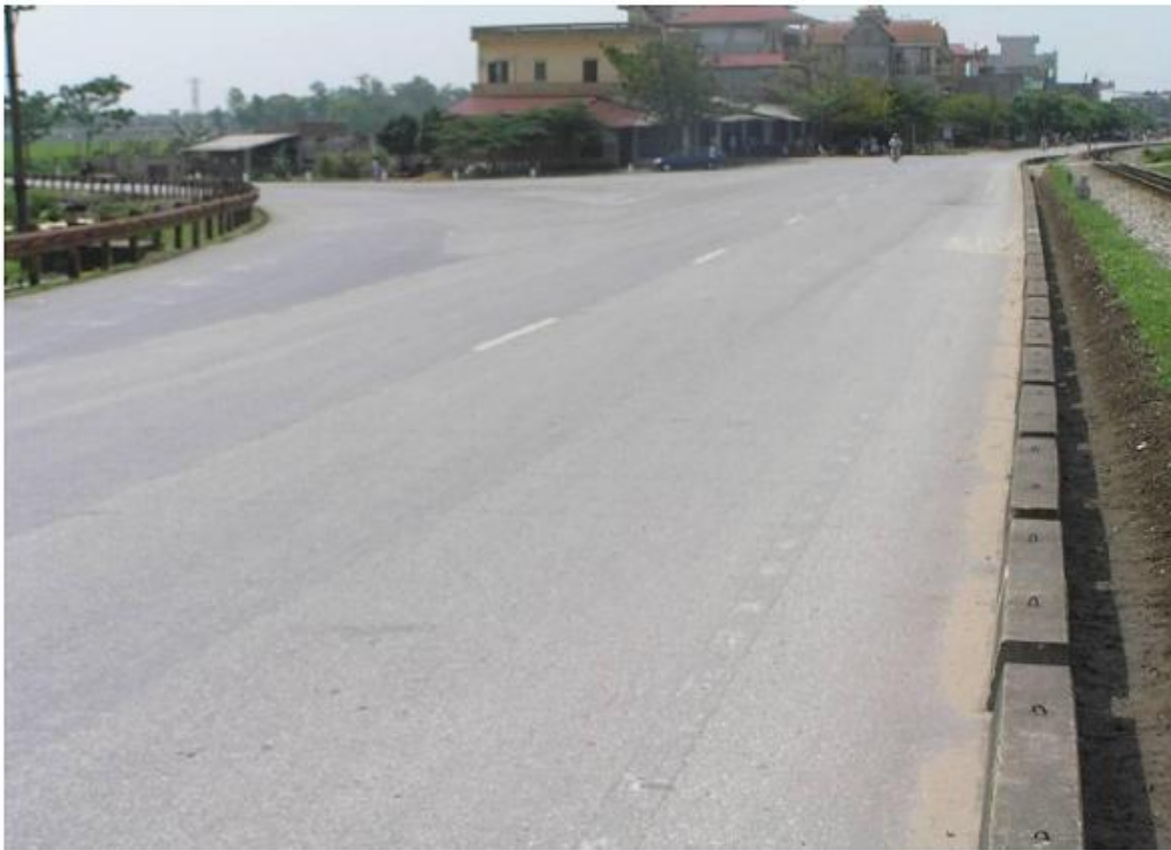
Figure 5: Excessively wide and open T-junction
