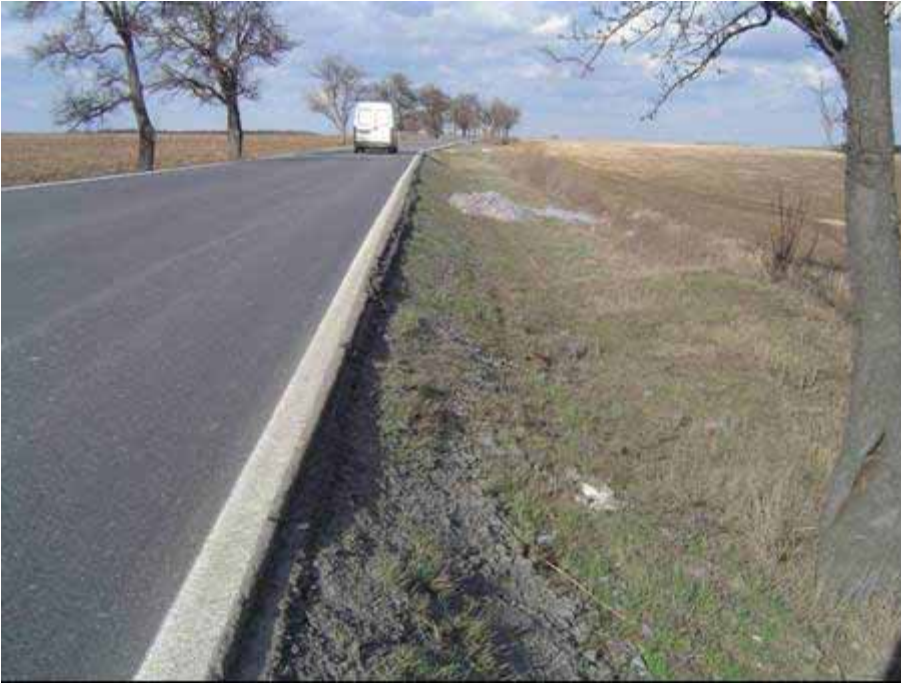
Figure 2. Lack of Roadside Shoulder along High-Volume Road in Suburb of Prague. 6
