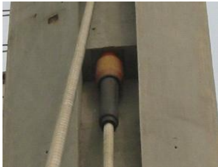
(a) Cable in service
