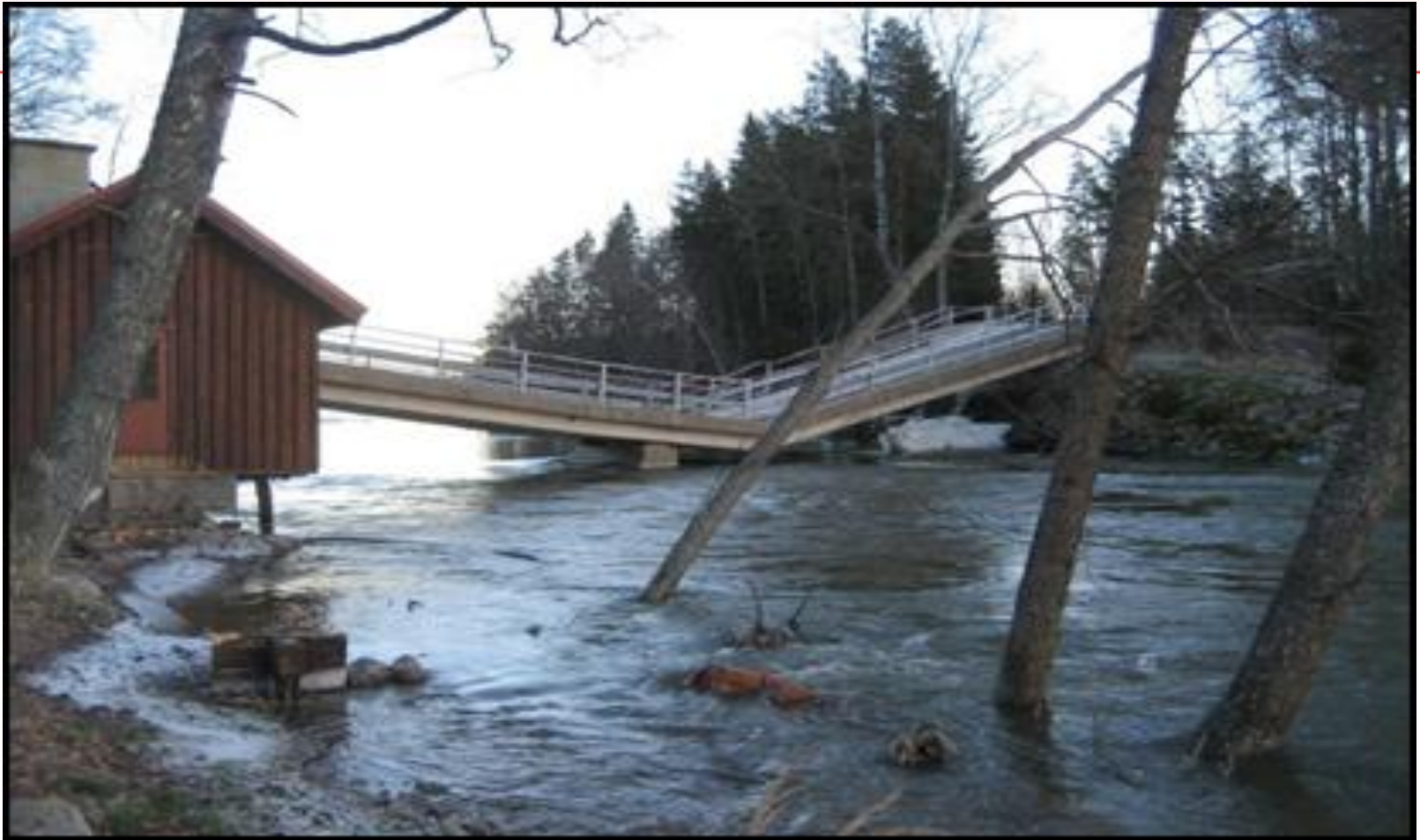
Collapse of a Bridge in Finland
