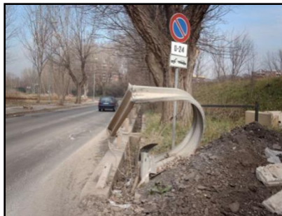
DEFORMED SAFETY BARRIER
