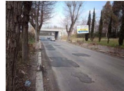
PATCH AND UNEVENNESS
