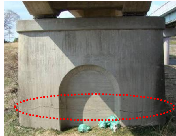
Damage to RC pier with small amount of reinforcement
