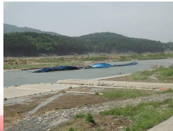
Steel girder washed away
