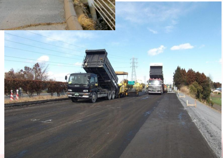
Subsidence of road embankment and temporary repair (Joban expressway)
