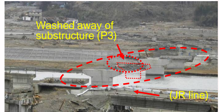
After earthquake (March 15)
