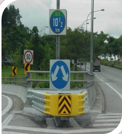
Installed crash cushion at hard gore area to save lives
