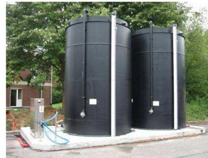
Brine tank facilities
