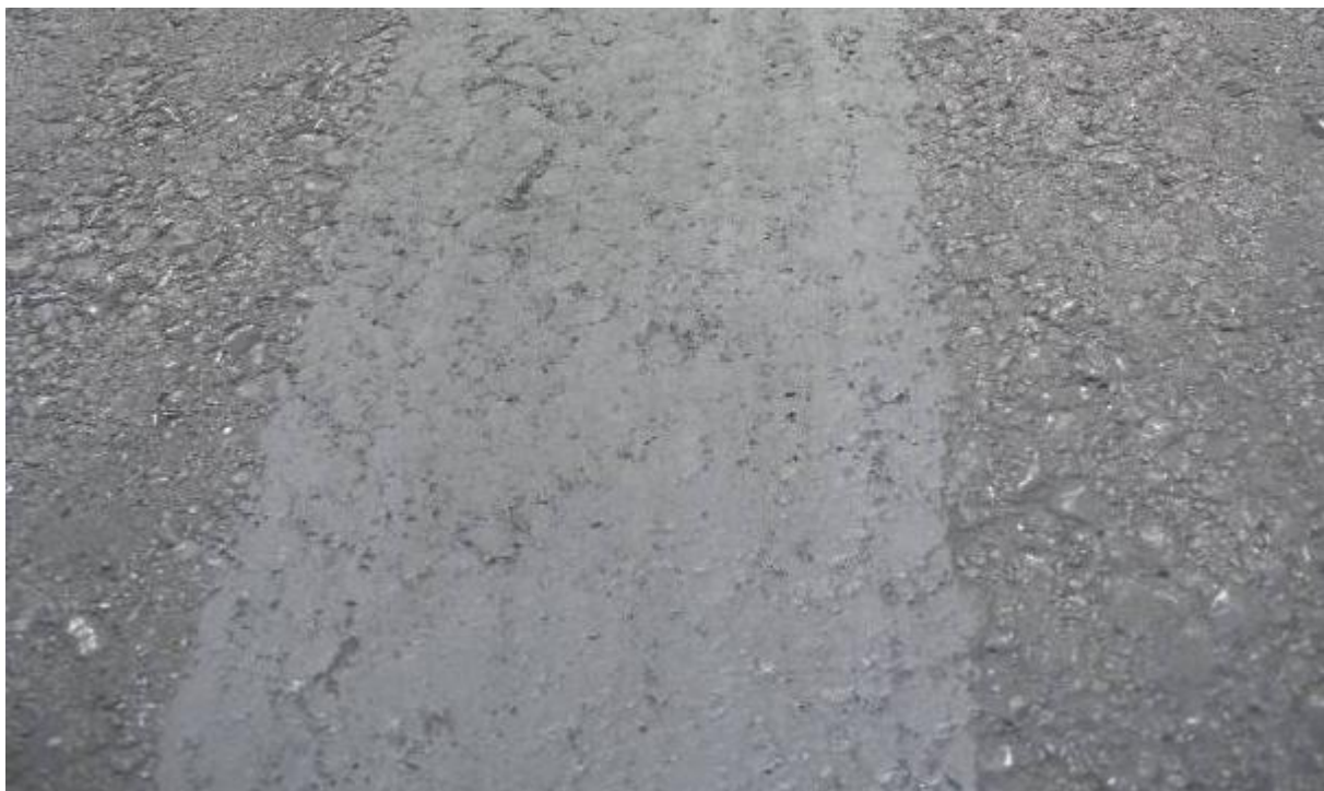
Figure 4 – close up detail of shiny wheeltracks on George 11/29 runway
