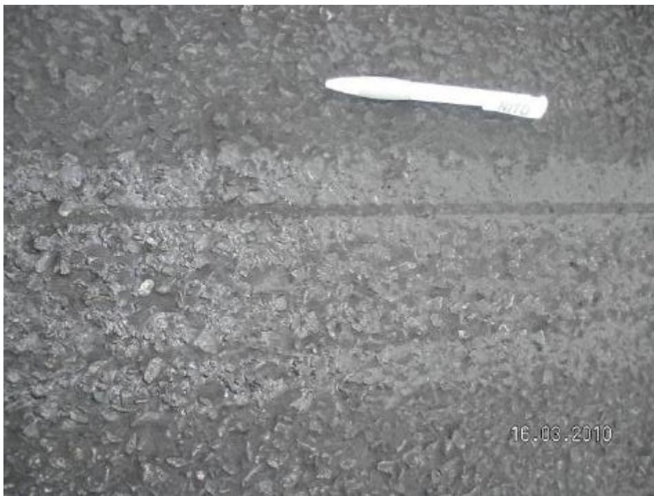
Figure 2 - Shiny wheeltrack, covered aggregate and filled-up voids
