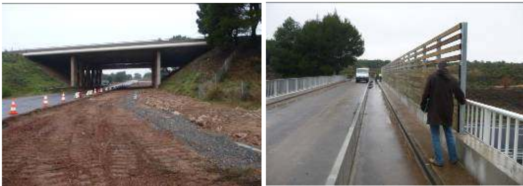
Figure 13 – Conversion work on an underpass (left) and an overpass (right) on the A9 motorway
