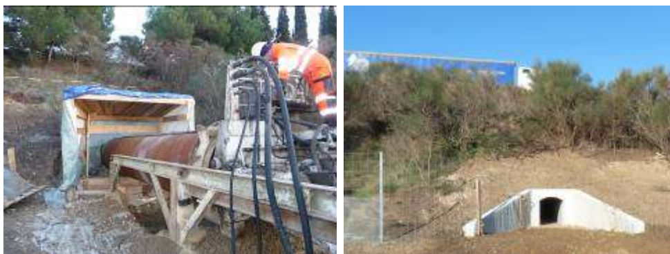
Figure 11 – Construction of a 1200 mm culvert (left) and finished structure (right) on the A7 motorway
