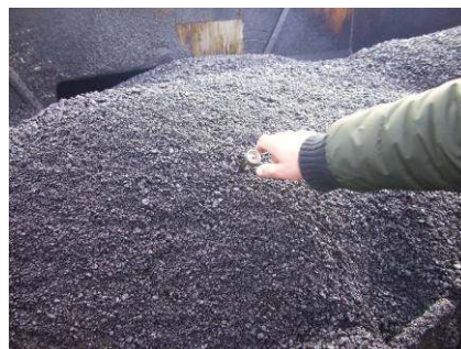
Figure 3 – Laying of the asphalt mixture; measuring the temperature of the asphalt mixture before laying and compacting.
