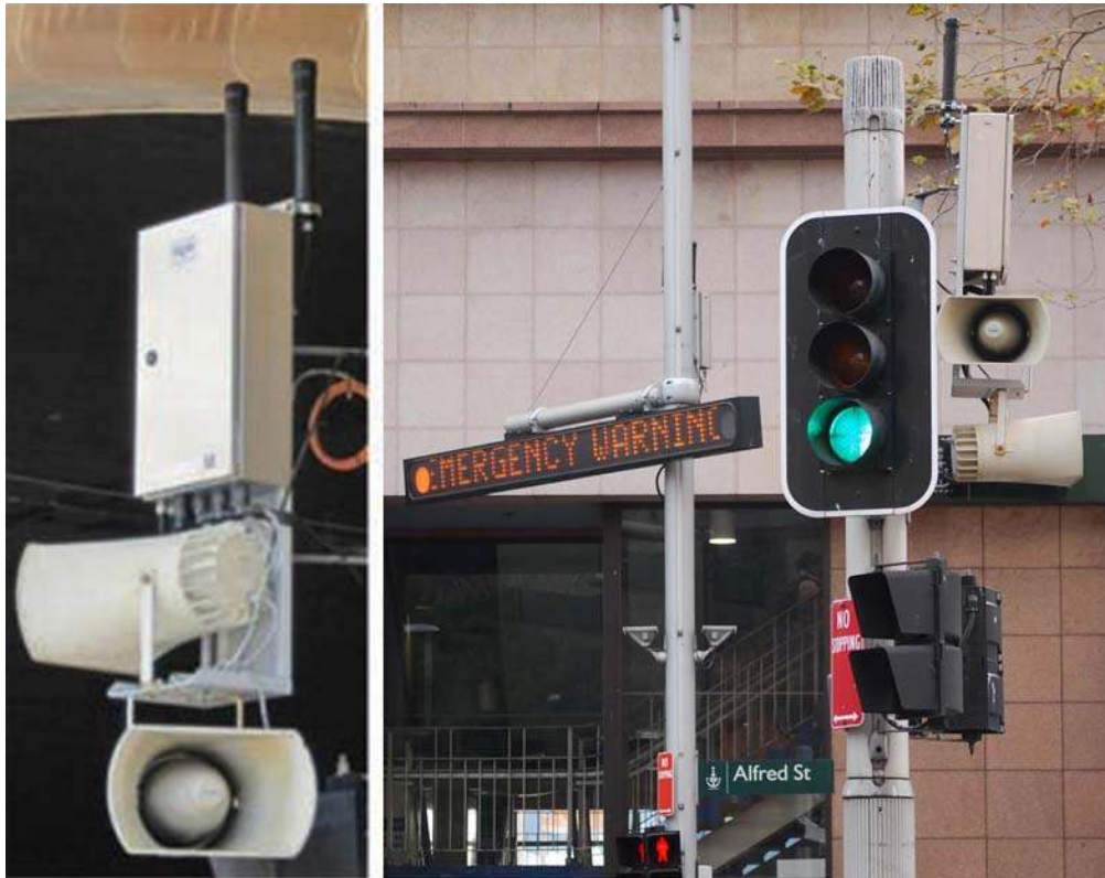
Figure 2 - Above left, speakers, control housing and aerials. Above right, single line scrolling Variable Message Sign, control housing and aerials.
