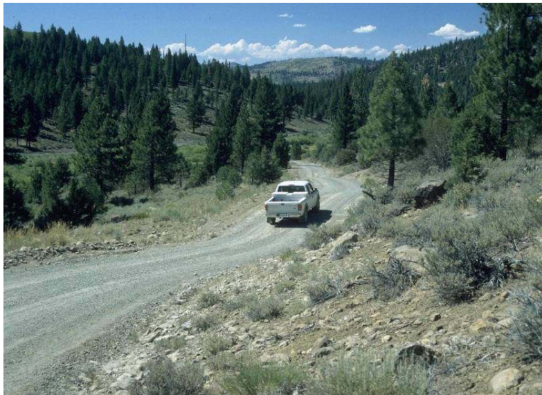
Figure 8 - A rolling dip cross-drain used to divert water off the road surface, as well as drain the ditch.
