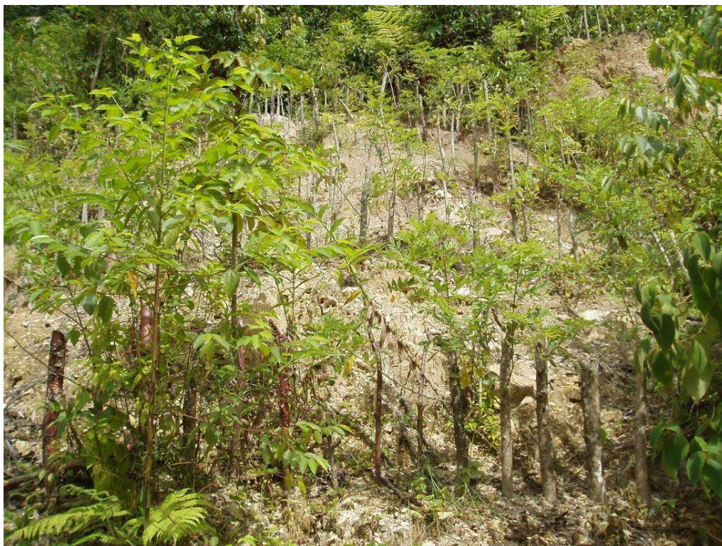
Figure 7 – Live stakes used in a shallow unstable area to help stabilize the landslide. Use plant types that grow deep roots!
