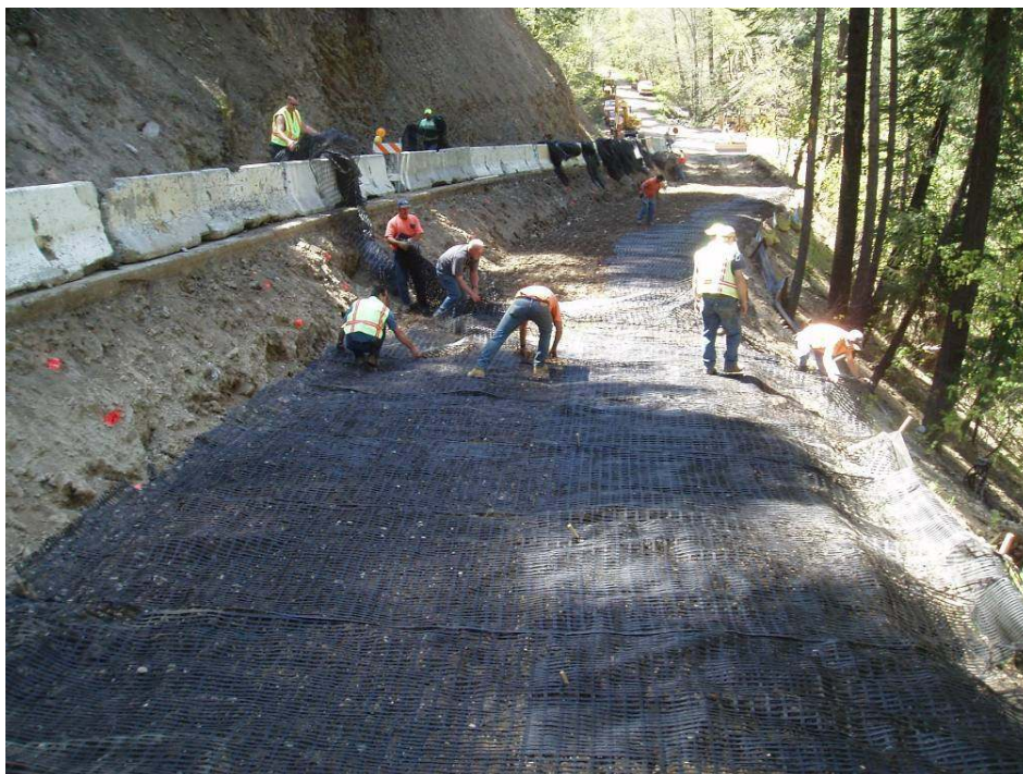
Figure 9 – A deep patch road shoulder repair using geogrid to reinforce a failing “sliver” fill slope.
