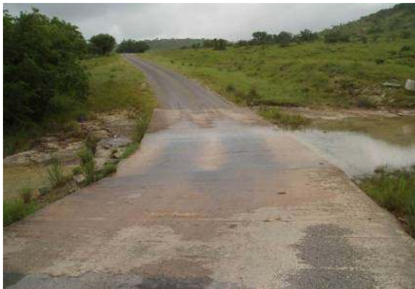
Figure 6 - A concrete slab low-water ford, with high flow capacity, used as an alternative to a large culvert or bridge.
