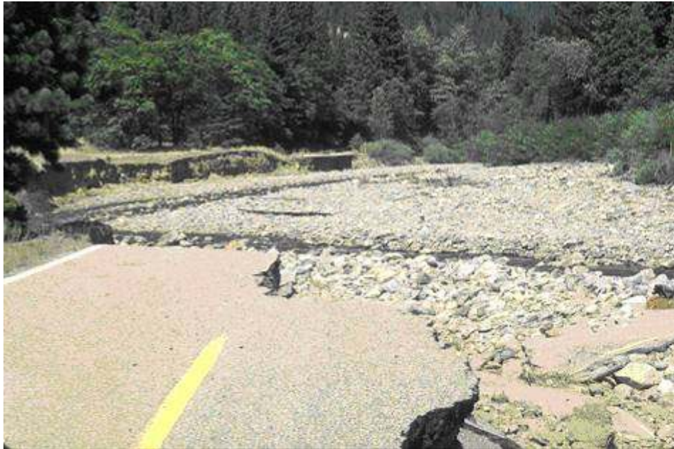
Figure 1 - A road washout due to poor road location on a floodplain.
