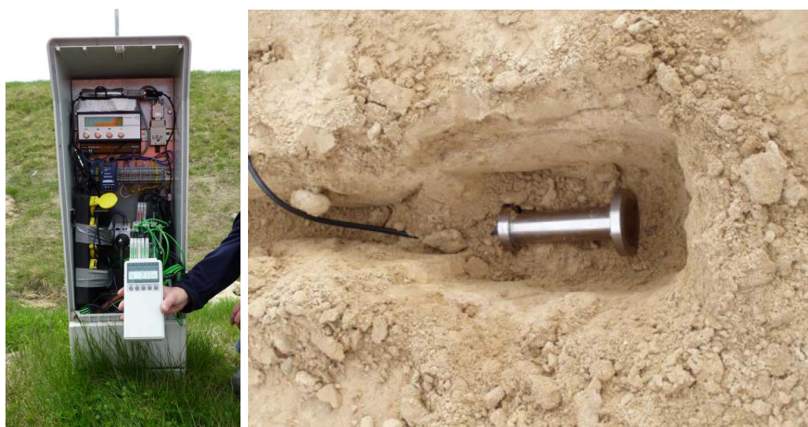
Figure 6 – Weatherproof cabinets for data logging (left) and moisture sensor (microwave head / right)
