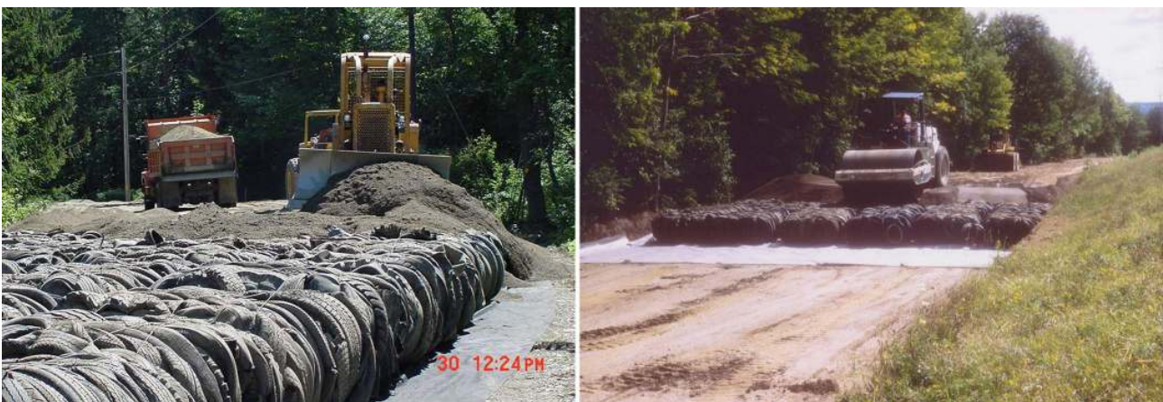
Figure 9 – Construction: bulldozing sand to fill voids, County Road 342 (CR342) in 2000 (left); vibrating sand into inter-bale voids, CR647 in 1999. (Photographs courtesy of Ken Smith, Chautauqua County Department of Public Facilities, New York State.)
