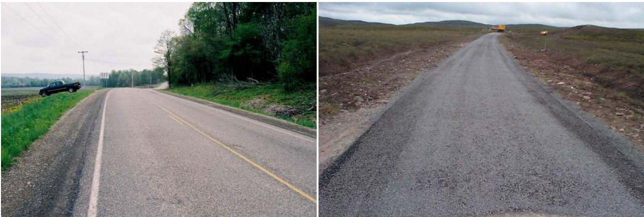
Figure 10 – Completed construction: CR342, May 2004 after four years in service (left); B871 in Highland, UK (right, photograph courtesy of Garry Smith, Highland Council).
