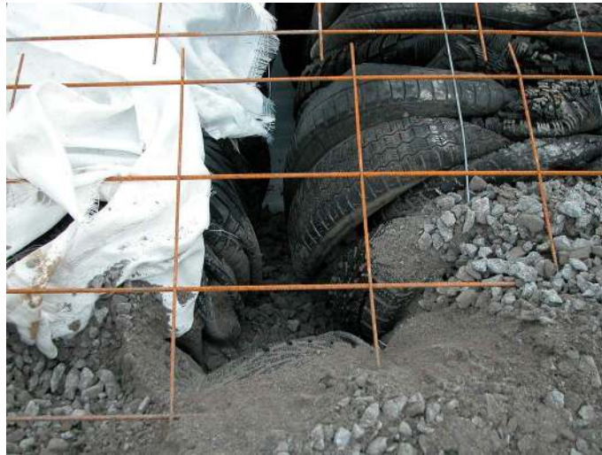
Figure 8 – Construction in which the bales have not been placed as close together as possible and in which the voids between the bales have not been well filled. (Photograph courtesy of Dennis Scott, Northern Tyre Recycling.)
