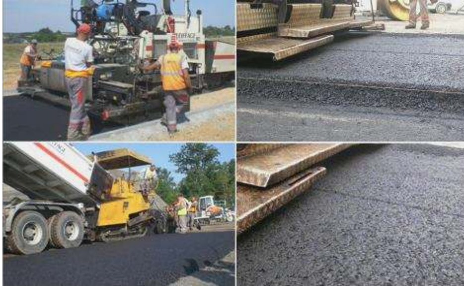
Figure 7 – Paving GB5 ® 0/14mm high-performance asphalt with Noubleau aggregates and 35/45B bitumen in the Tours area. In-place density: 96.4% ; stiffness modulus measured in indirect tension configuration E^*(15^{\circ}\text{C}-10\text{Hz}) : 14,100MPa.
