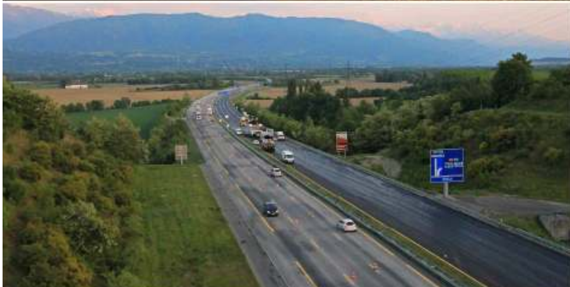
Figure 9 – 12 000-ton GB5 ® 0/14 roadwork on the French A43 toll highway (AREA network, Chignin-Francin section) in the alpine area. SBS-modified binder Biprene ® was used.
