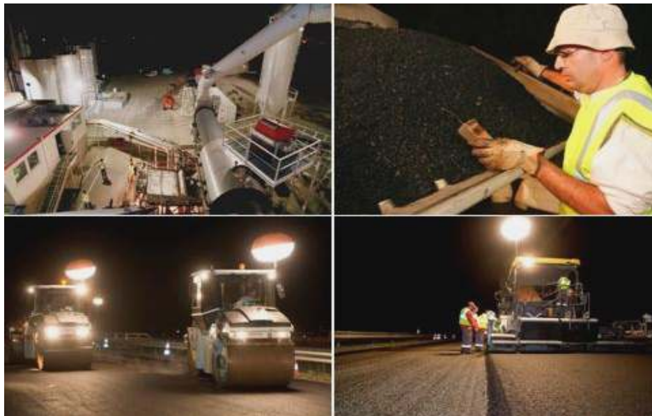
Figure 8 – Paving GB5 ® 0/14mm high-performance asphalt with Cemex aggregates and 35/45B bitumen and 35% RAP (reclaimed asphalt pavement) near Toulouse. In-place density: 97% ; stiffness modulus in indirect tension mode E^*(15^{\circ}\text{C}-10\text{Hz}) : 15,100MPa.
