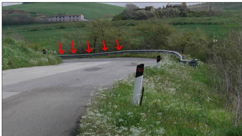
Figure 2 - Extensive subsiding of the outer edge on a bend with escarpment (high hazard level)
