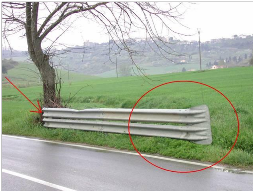
“Figure 5 - Unprotected tree, inadequate protection of the ditch (high hazard level)”!
