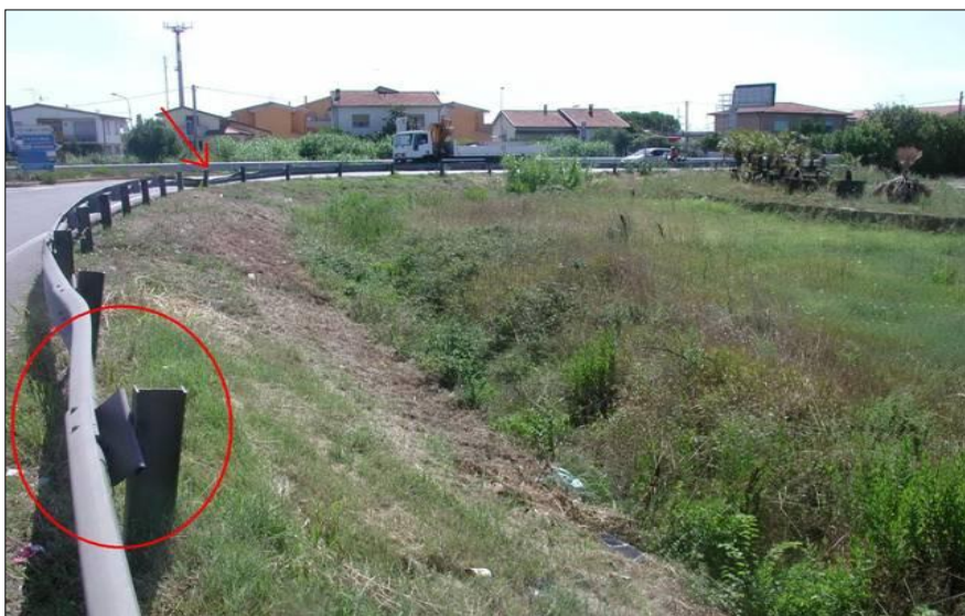
Figure 3 - Detached guardrails and deformed spacers (medium hazard level)
