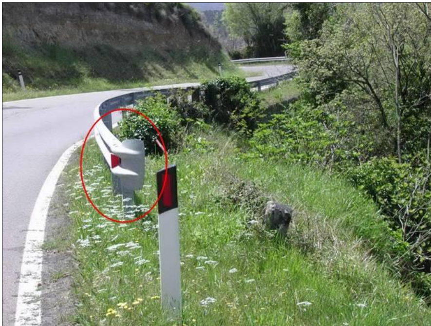
Figure 6 - Inadequate guardrail terminal end (high hazard level)
