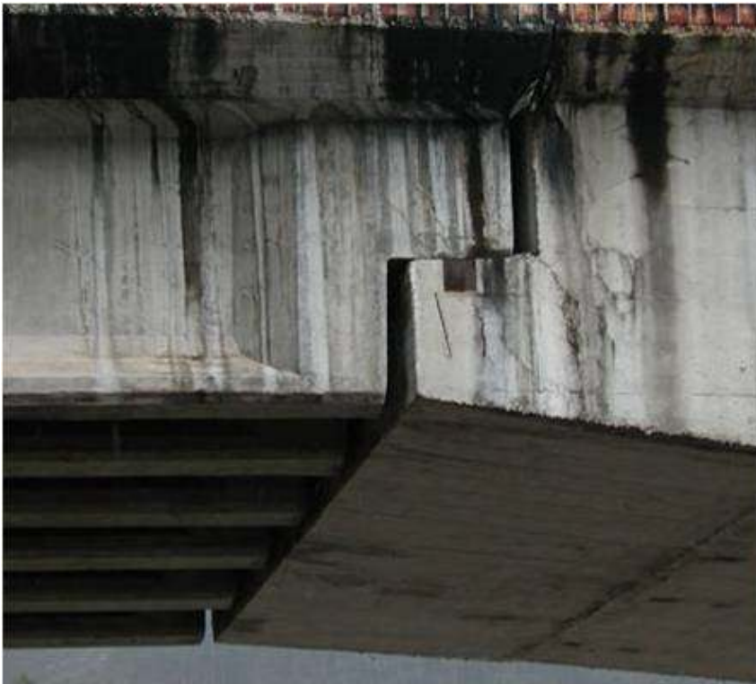
Figure 8. Example of intermediate support, with great difficulty of inspection.
