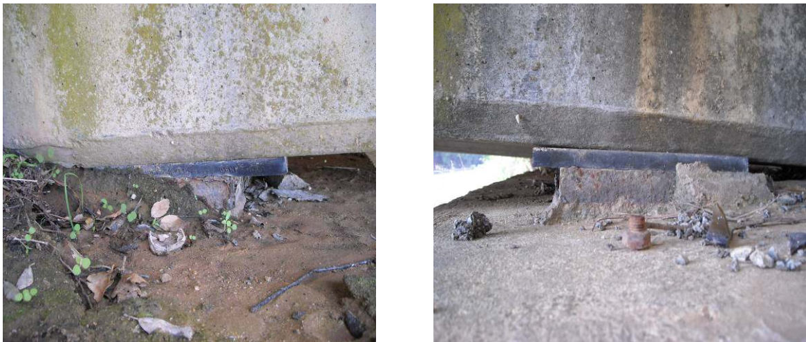
Figure 5 – Blocked bearings o out of place
