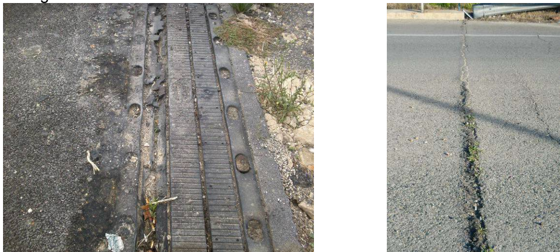
Figure 6 – Damaged expansion joint . Non existing expansion joint
