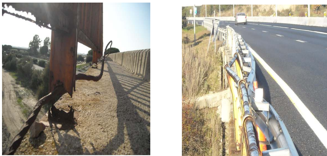
Figure 7 – Damages on steel guardrails and barriers
