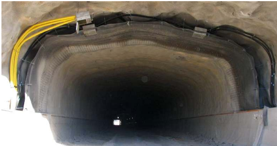
Figure 2 - Typical water and frost insulation lining structure from a Highway 1 motorway tunnel in Finland. Polyethylene sheets are installed with steel bars and steel net, and fire protected with schotcrete. There is minimum 250 mm of empty space behind the lining.
