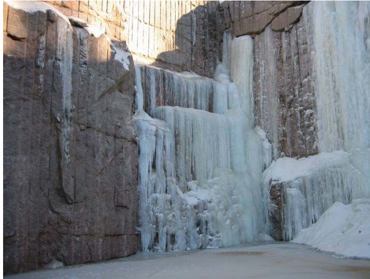
Figure 1 - Frozen ground water leakage from a rock joint in a construction phase for motorway tunnel entrance on Highway 1, Finland.
