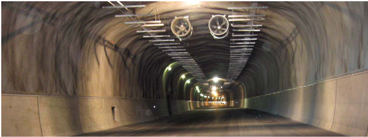
Figure 3 - Ready made interior in a motorway tunnel. Final lighting to be installed.
