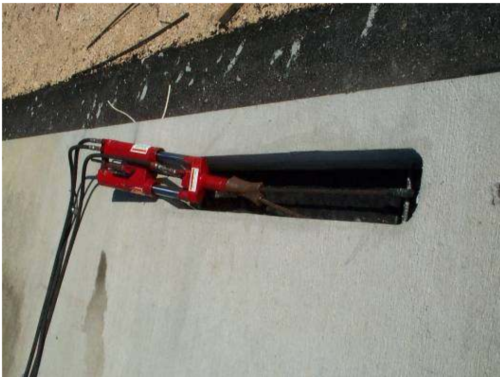
Figure 7 – Stage I stressing at central stressing pocket.
