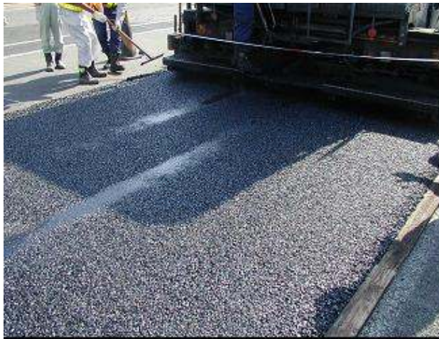
Photo 6 - Bitumen's run-off problems [8]
