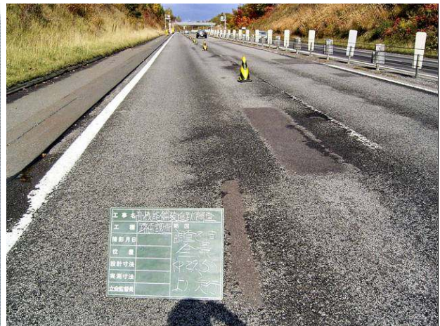
Photo 4 - Severely abraded road surface
