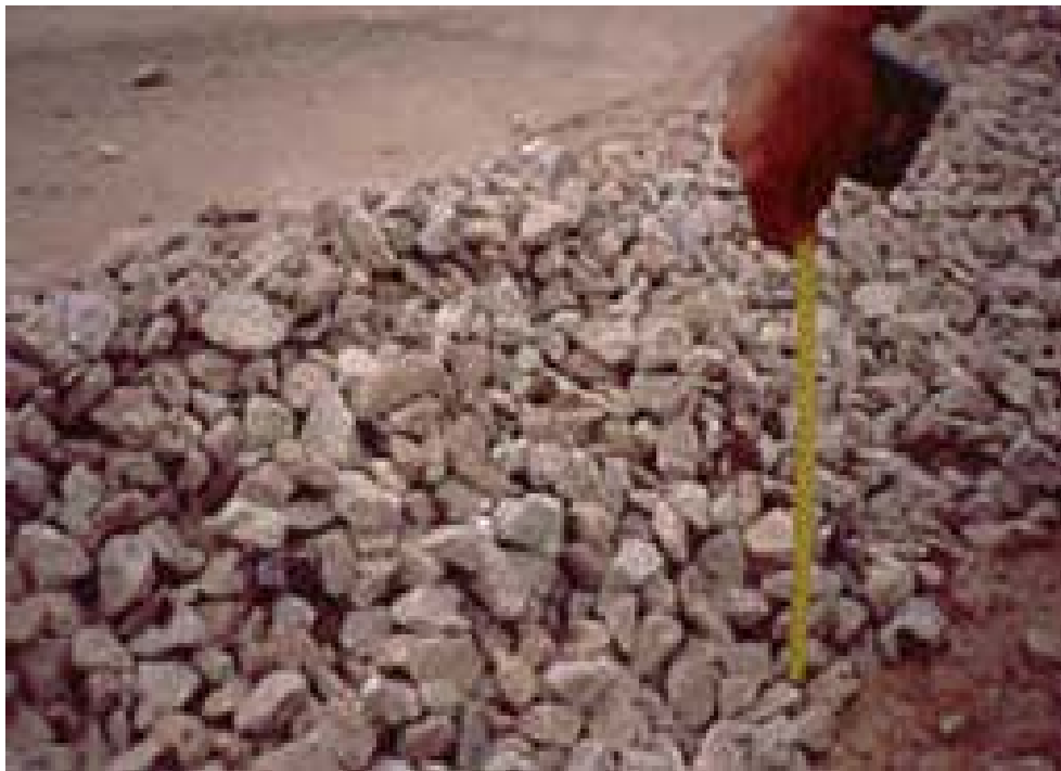
Figure 4 - "Inverted section pavement Durango airport. Surface course: 15 cm; base course: 40 cm; sub-base course: 30 cm.
