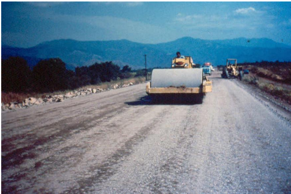
Figure 14 - CCR compaction (sub-base course) of “inverted section” pavement. Tepic – Aguamilpa highway. Portland cement content: 10%; thickness: 25 cm. Alluvium gravel.
