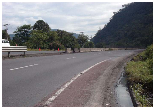
FIGURE 5 Condition of the central barrier in Segment 4
