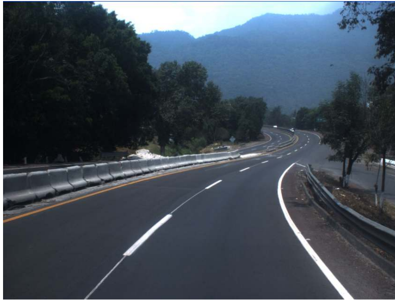
FIGURE 2 Discontinuous concrete central barrier in Segment 1
