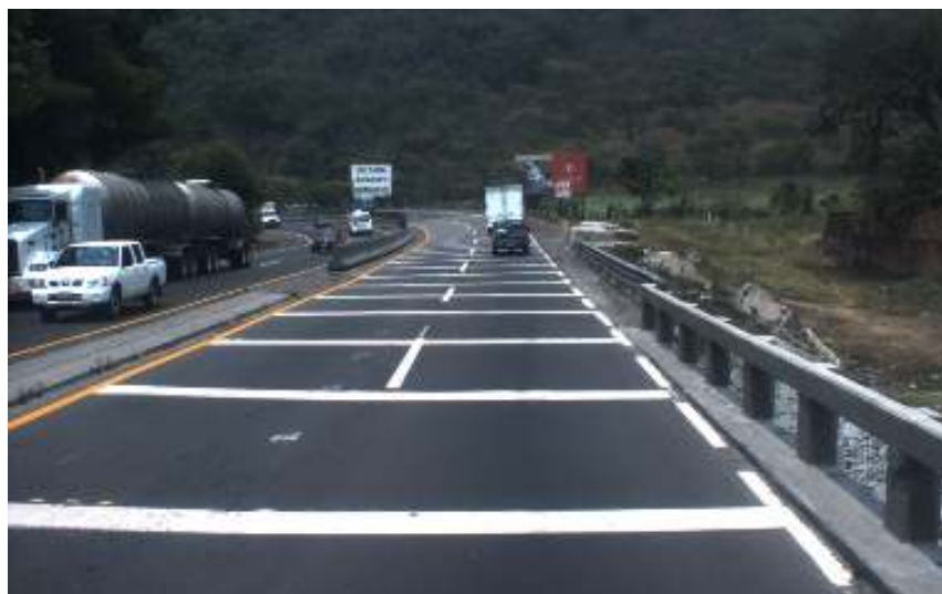
FIGURE 3 Reduction in the cross section of the bridge at Segment 2
