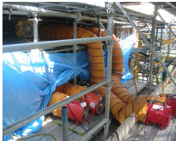
Photo 1 - View of air cooling
