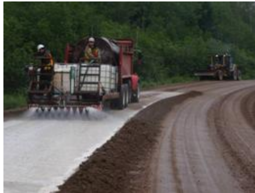
Figure 6 – Spreading of the stabilization agent at 5 cm deep on the left side of the road
