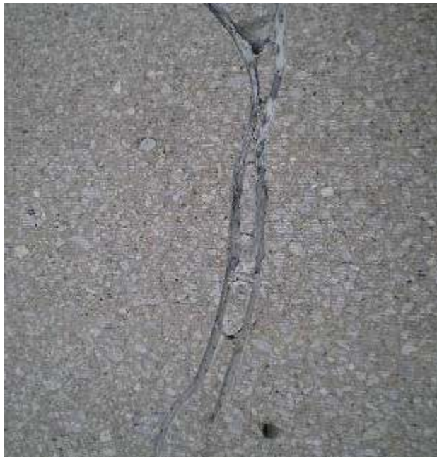
FIGURE 4. Cracking at a stitch that was completed too late.
