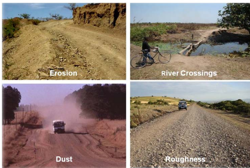
Figure 2 - Typical problems on gravel road networks
