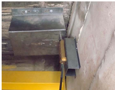
Figure 5 - Optical strain gauge installed on bearings
