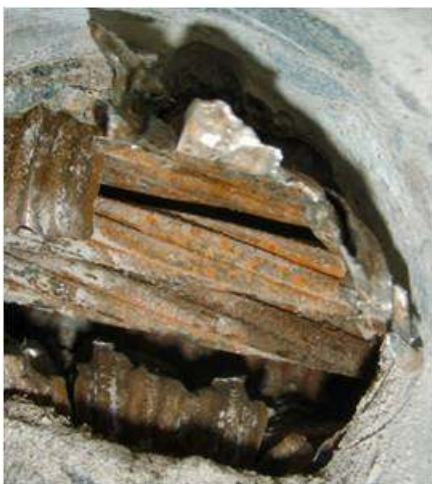
"Figure 8 – Exposed prestressing steel, drilling location in accordance to 3D TOMOGRAPHER scanning"
