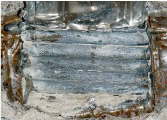
“Figure 11 – Exposed prestressing steel, drilling location in accordance to 3D TOMOGRAPHER scanning”
