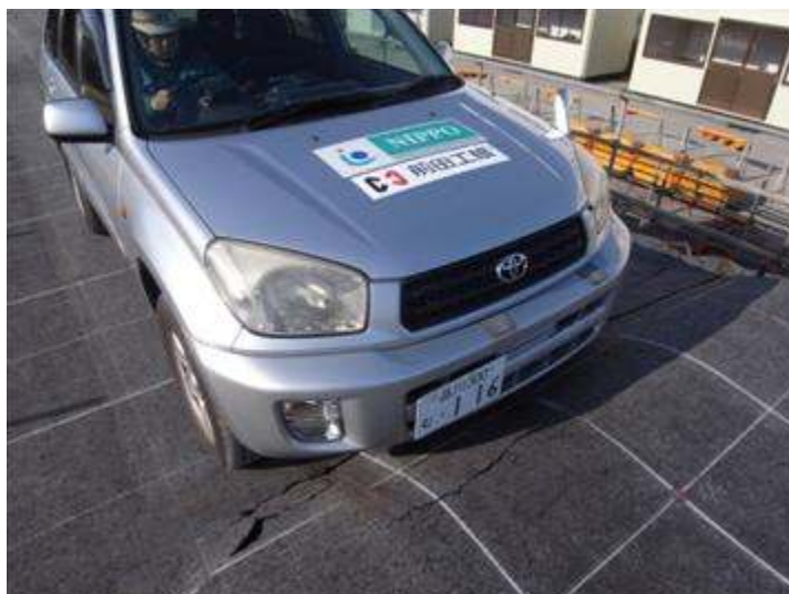
Photograph 16 - Trafficability tests on asphalt pavement on normal subgrade after 300mm forced settlement
