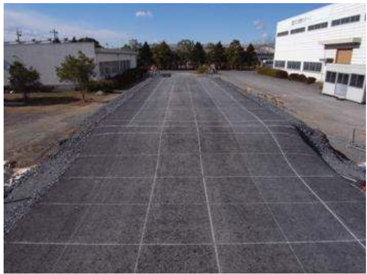
Photograph 13 - Deformation of asphalt pavement on CRE after 300mm forced settlement
