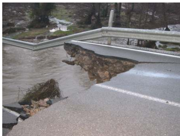
Figure 1 - Road failures in Sardinia caused by intense precipitation (photos by ANAS)
