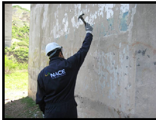
Figure 3 Detection of hidden corrosion in pile 3 Mezcala Bridge
