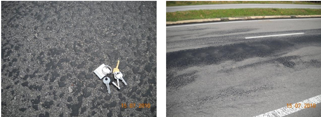
Figure 2 - Bleeding at newly constructed Lebu AMJ
