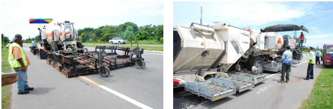
Figure 6 - Pre Heater and Remixer
