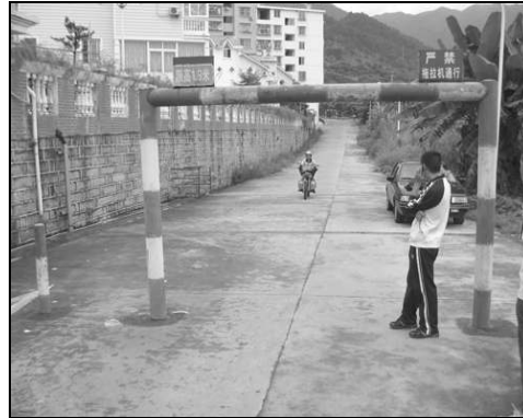
Figure 7 - Unsafe pillars of height restriction barriers
