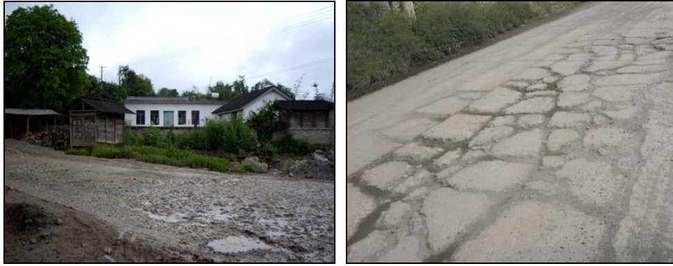
Figure 1 -Village road destroyed by overload trucks
