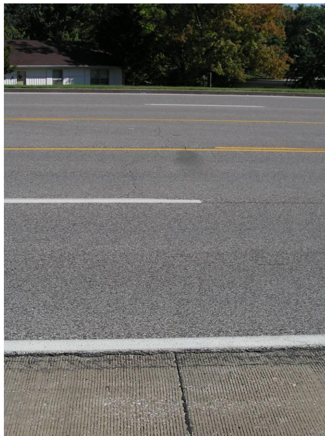
Cracking in Center Lanes of Lindbergh, 2008
