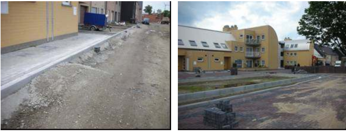
Figure 11 – Temporary structure to provide entrance to the houses and view of the final work site in Sint-Niklaas, Belgium.
