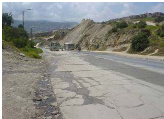
Picture 2. Road deteriorated due to groundwater Usme; Colombia
