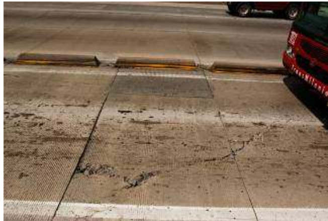
Picture 1. Transmilenio slab damage on North highway; Bogotá Colombia
