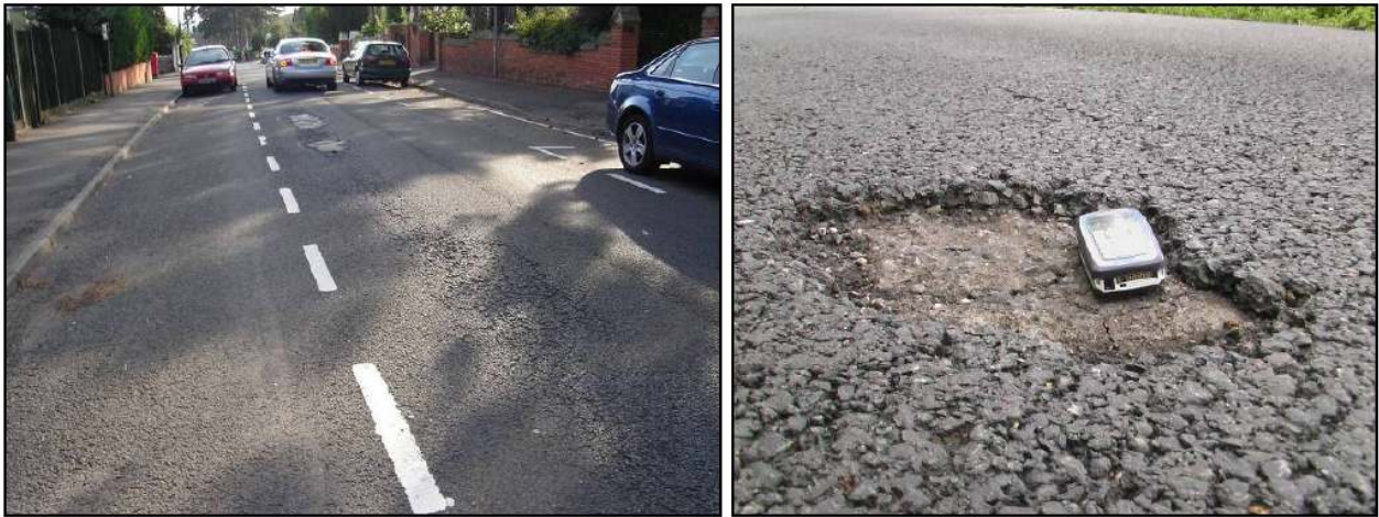
Figure 4. Two of the most common problems with TAL: ravelling (left) and delamination (right). Photo courtesy of Ian Walsh, Jacobs Engineering (UK) Ltd.
