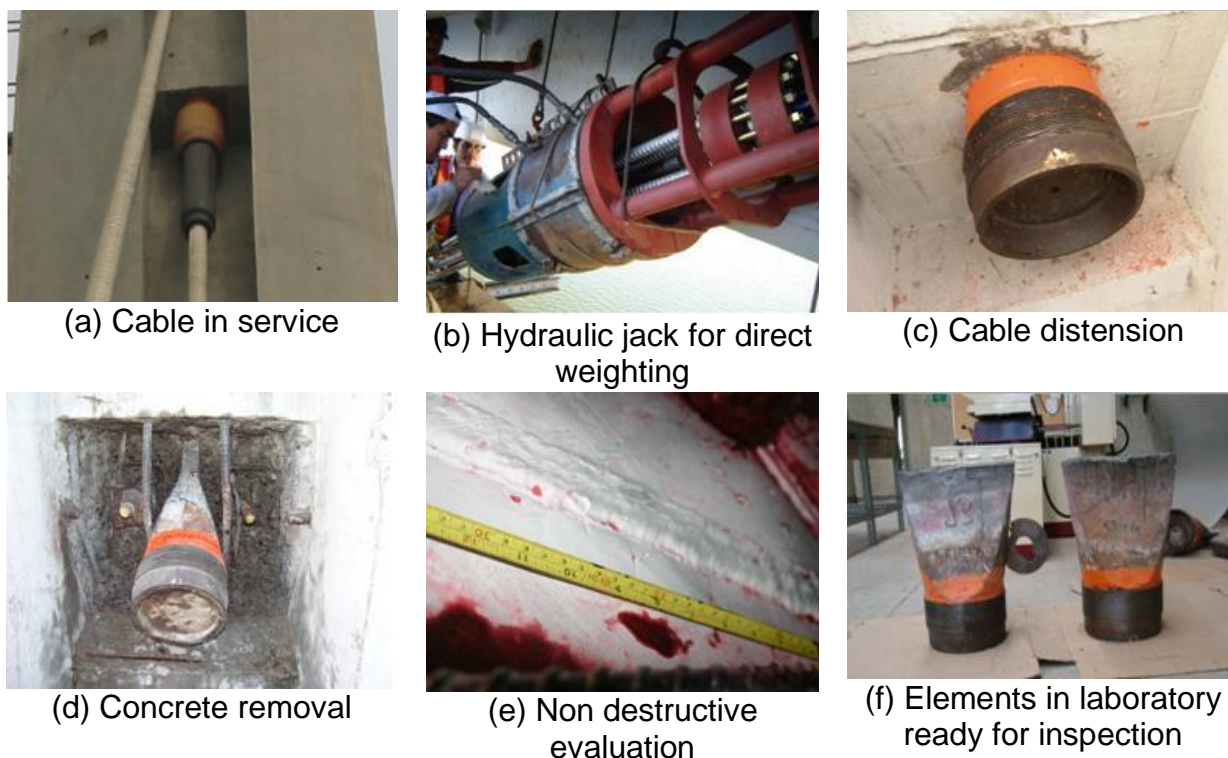
Figure 13 - Pictures showing the general process used for the rehabilitation of the upper anchorage elements.
