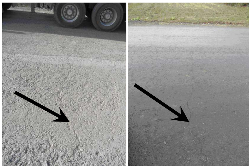
Figure 5 – Characteristic transverse crack on the recycled course (left) and asphalt course (right)
