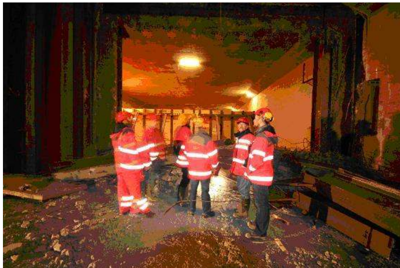
Figure 3 - A site visit to the Opera Tunnel under construction (Kjell Solem, NPRA)
