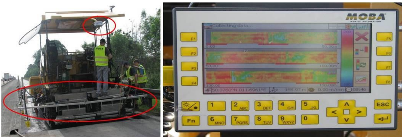
Figure 8 – Positioning of the temperature measurement devices on the asphalt paver (left), display unit on the asphalt paver to monitor and document asphalt mixture temperatures during installation (right)
