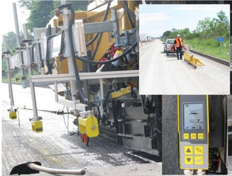
Figure 10 – “Big-Sonic-Ski” mounted on the research paver, electronic display unit and automated control unit as well as planograph measurements
