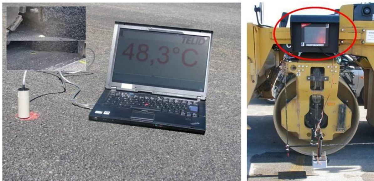
Figure 9 – Installation of passive temperature sensors and reading of the current asphalt temperature in the installed layer (left) and the temperature display unit on the roller (right)
