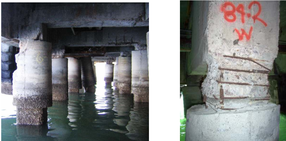
Figure 2- Incorrect repairing of a corroded pile on the North and South Pier respectively.
