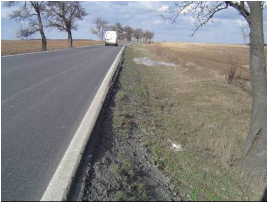
Figure 18: Completely missing shoulder along the busy road in Prague suburb
