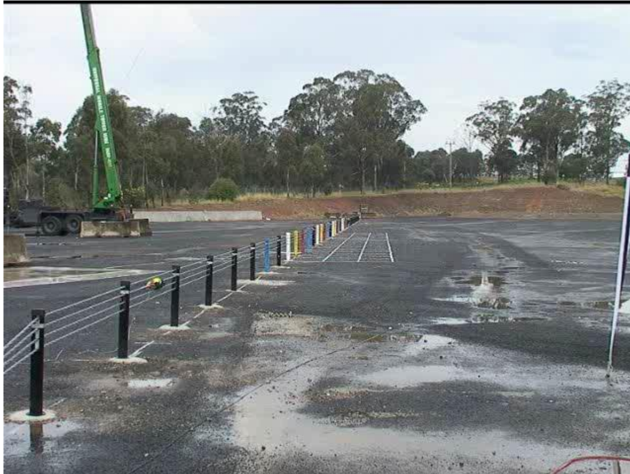
Wire Rope Barrier
