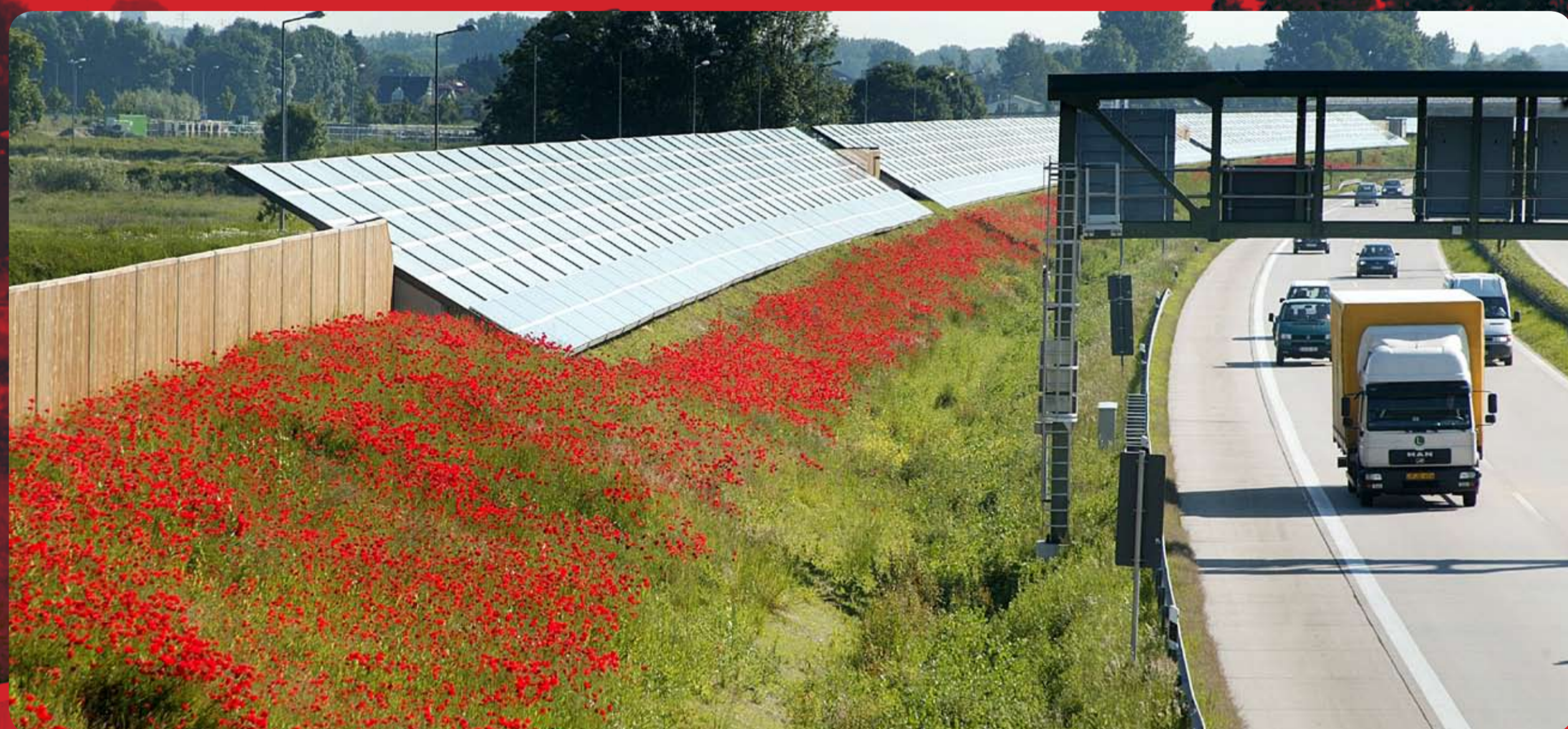
Photovoltaic panels on noise barriers to use renewable energy sources (PV-Soundless, Noise Barrier, EU-Project)
