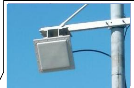
ITS Spot Unit (roadside unit)
